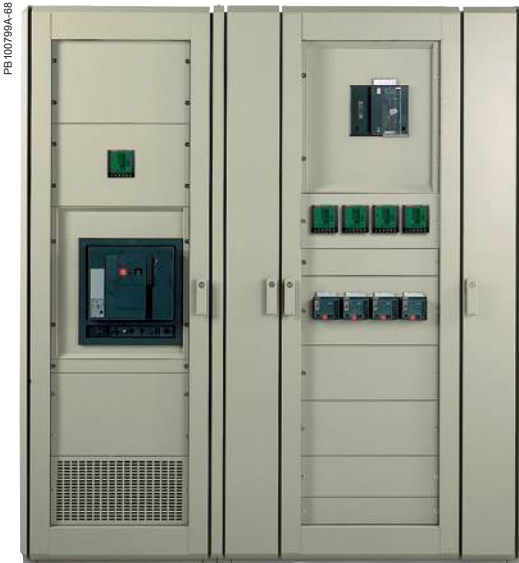
Main LV switchboard.
